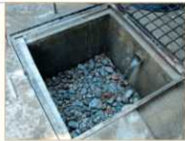
RAINWATER HARVESTING PIT
